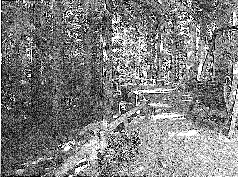
Photograph 6. View of fill and wooden retaining wall extending into parklands on Lot 1.
